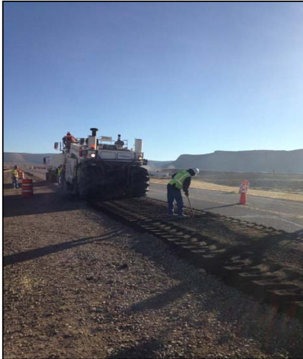
Full depth reclamation of existing road on the Trail of the Ancients
